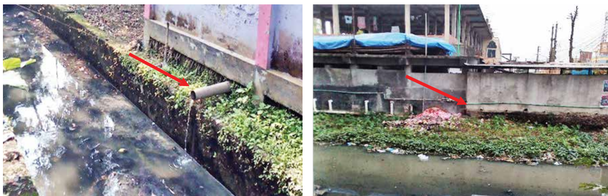
Figure 6: Containment technologies and their connections in Barishal. Left: Toilet Pit open to a nearby water body, Right: Toilet pipe connected to open environment (Source: Feasibility Study 2020-21/DPHE)
